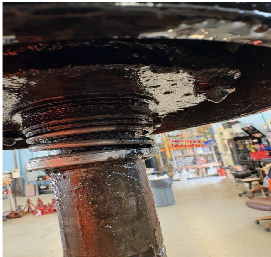
NWLS LF Pump 1 – Failed shaft seal (above).
