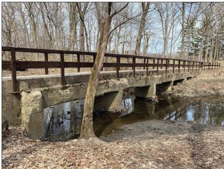
Photo of the bridge in its current state, courtesy of the Forest Preserve District of DuPage County.
