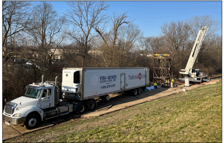
‘Cured in Place Pipe’ technique being used for the Curtiss Street trunk sewer rehabilitation project. Photo courtesy of Visu-Sewer, LLC.
